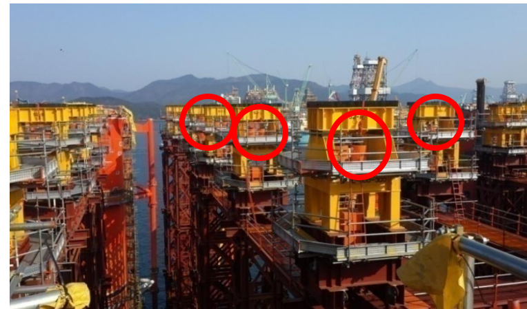
The whole view of installation
