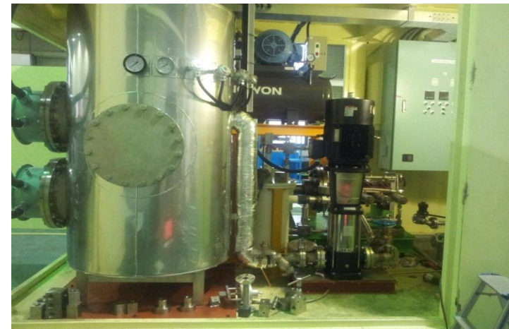
Inside of the equipment
